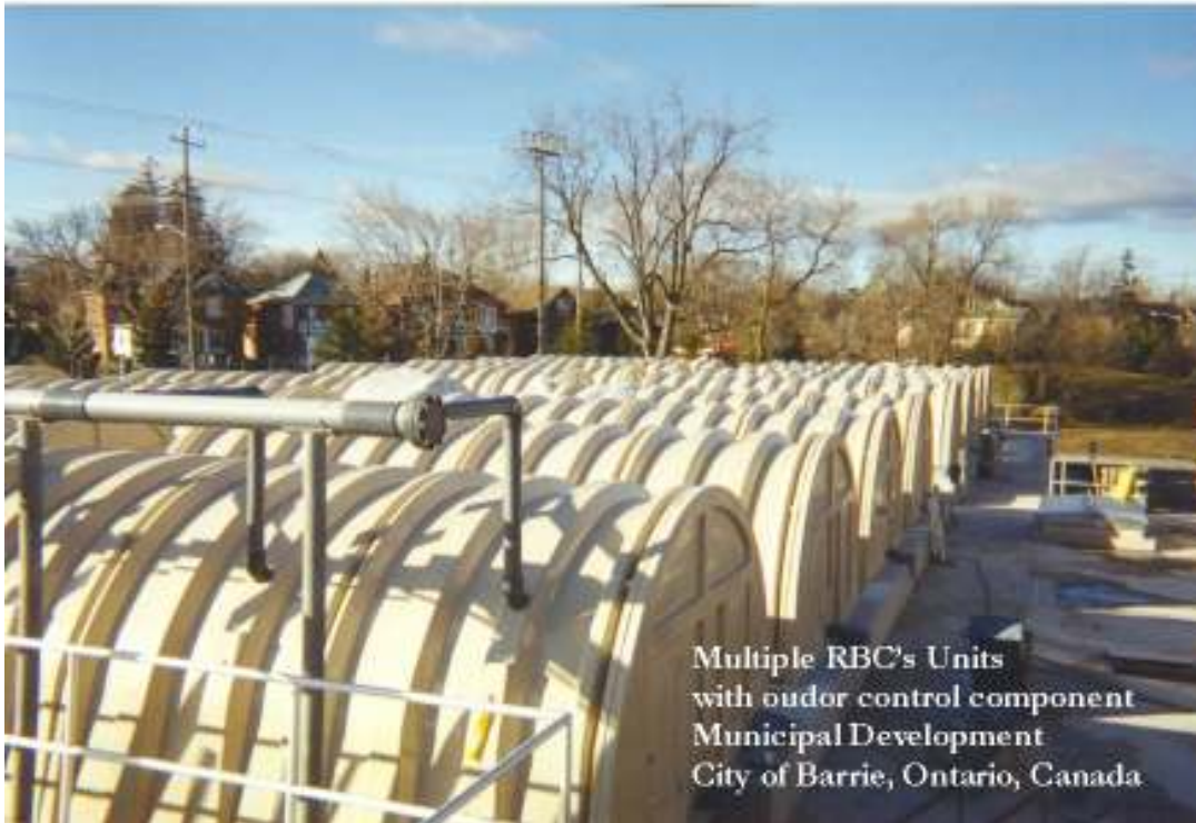
City of Barrie: Municipal Tertiary Wastewater Treatment Plant
